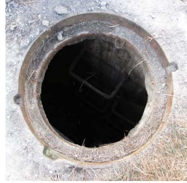
Effluent bypass canal
