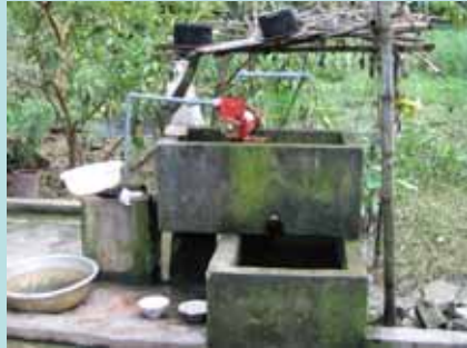
on the ground and electric pump
