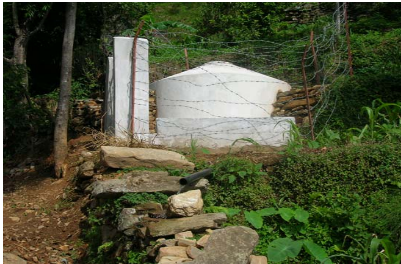
Reservoir Tank (RVT)
