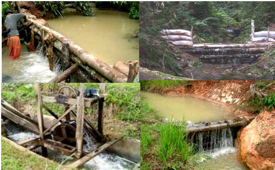
Figure 3. Simple check dams to reduce sediment load and flow velocity. Some of the water is used for micro hydropower station
